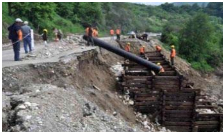
Fig.3. Landslide on Vaziani-Gombori-Telavi (Georgia) motor-way
