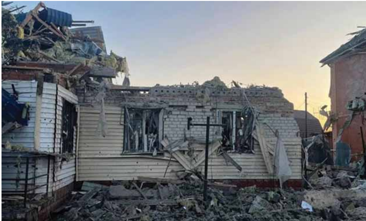
Damaged house following what Russian authorities called a Ukrainian military strike on the town of Sudzha. REUTERS
