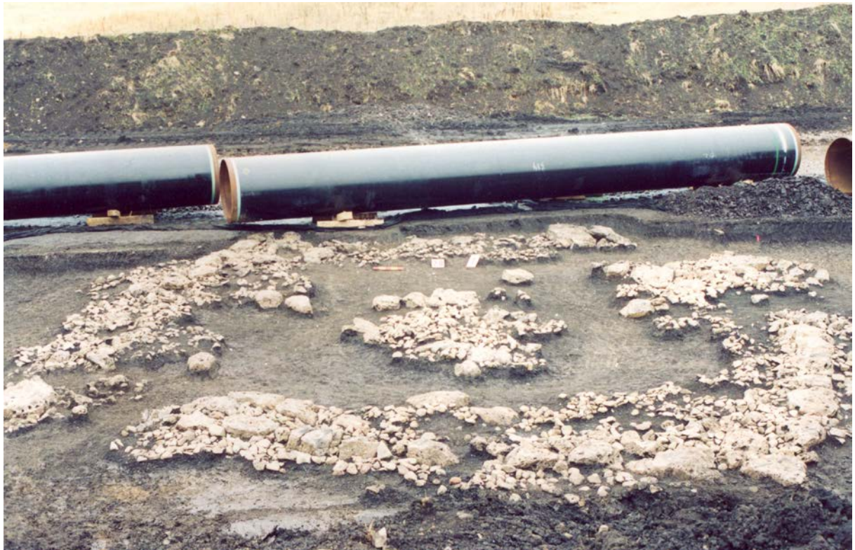
Fig. 224. Burial No. 20. The view of the mound damaged during construction works within the energy corridor after preparation.
