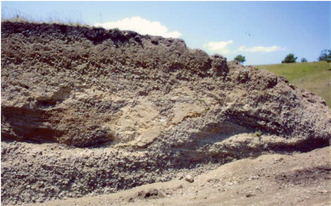
Pic. 328. Tsintskaro. Palaeontological monument, damaged while widening the road.
