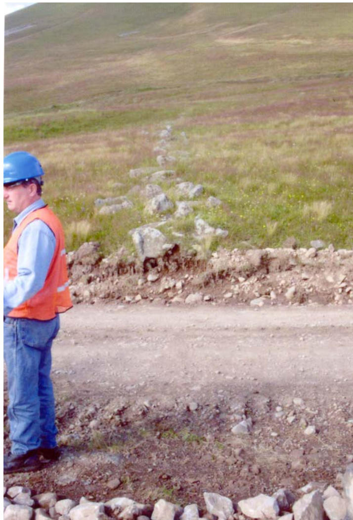
Pic. 353. Sapitiakhsho. The wall damaged during road construction
