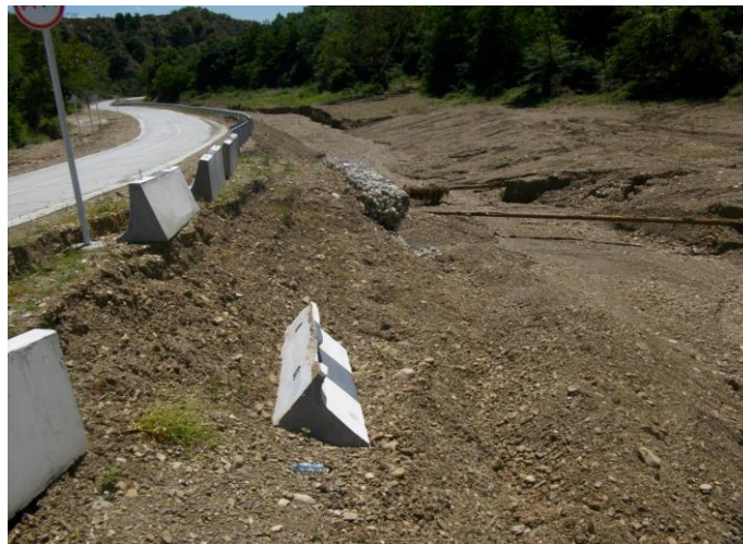
Picture 3. Damaged embankment of highway - stone pile gabion
