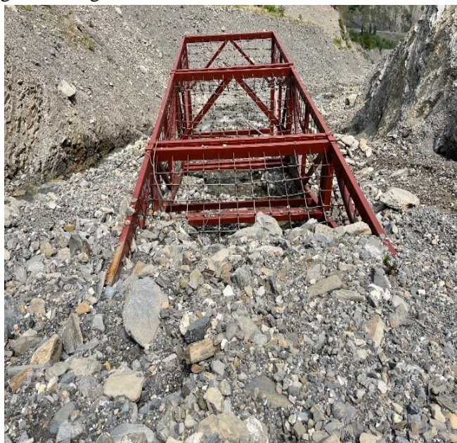
View of the structure after the debris flow passage
