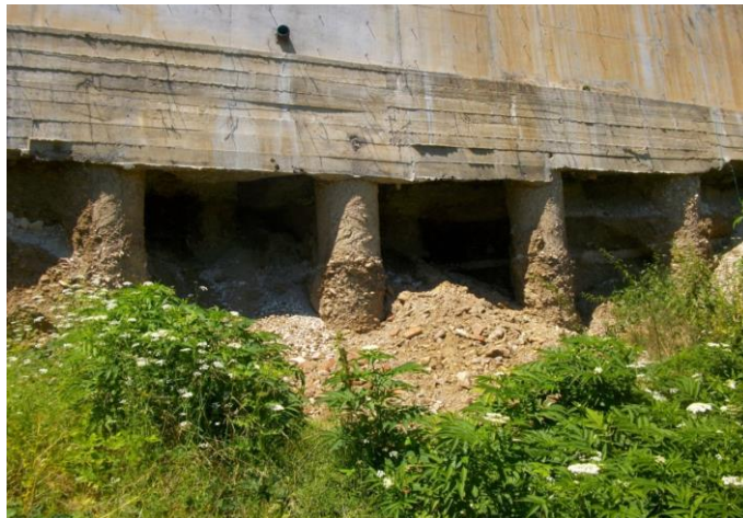
Picture 2. The damaged bypass at the back of the monastery
