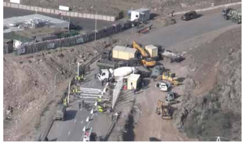
Azerbaijani construction crews building the checkpoint (center) with the Russian military base nearby (top left). Source: RFE/RL video
