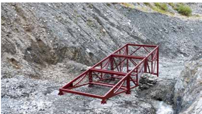
Debris flow elastic barrage in the bed of the Mleti river gorge (October 8, 2022)
