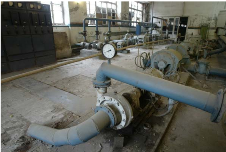
Fig. 2. The pumping station
