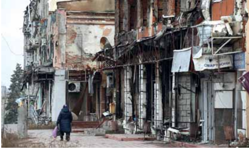
A local resident walks past heavily damaged buildings in the town of Izyum, Kharkiv region, on November 25. Photo by Anatolii Stepanov/AFP/Getty Images
