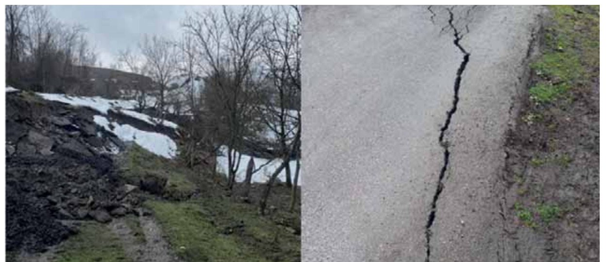
Collapsed and cracked roads in Itkhvisi. FB / Giorgi Makhatadze
