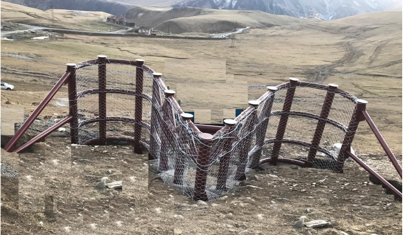
Photo. 4.1. An Overview of Innovative Snow Avalanche Construction Georgian Military Road in Kobi-Gudauri alpine zone (2238 m above sea level)
