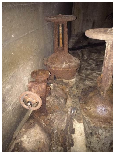
Fig. 2. The condition of the pipeline of reservoir depletion and the regulating closures on it
