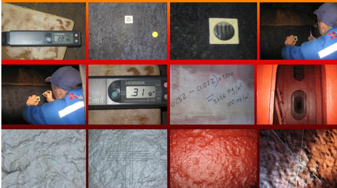
ISO 2409 Adhesion 1 point ASTM D 3359 Adhesion 5A Reading before application of “CONTRRUST” - 22 points, after – 0.31 point
