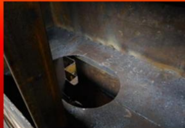
Surface condition is «D» in accordance with ISO 8501-1
