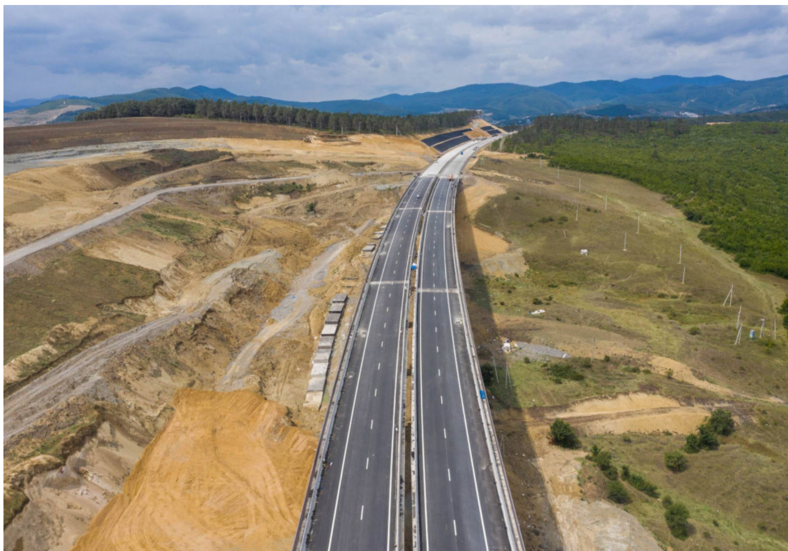
► The construction of the Khashuri bypass road, which is part of the East-West Expressway (E60) as part of the Upper Osiauri-Chumateteli project, is nearing completion.
