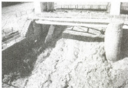
Photo 2. Damaged Khoni-Martvili vehicle bridge and adjacent meliorate head building by the Tskhenistskali River flood
