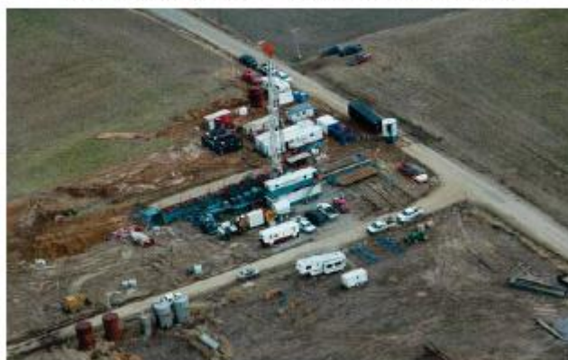
MPD Surface Equipment Setup (Well No. 2)
