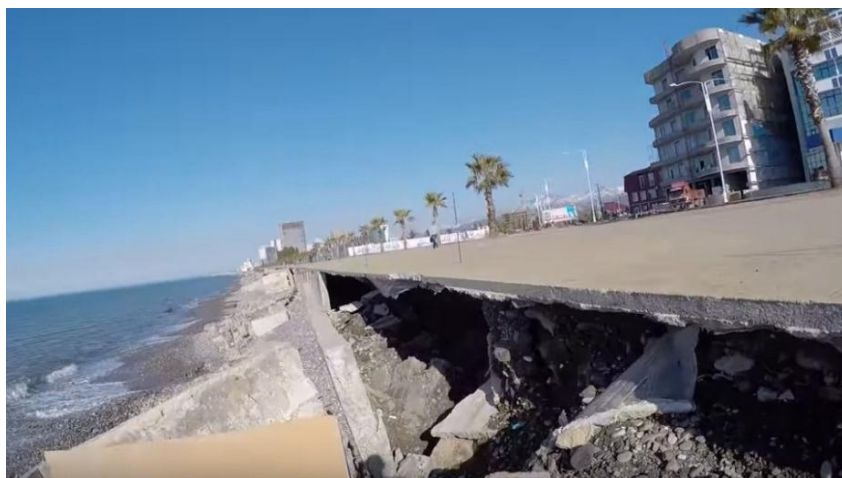
Fig. 4. Collapsed promenade near Adlia (2016)
