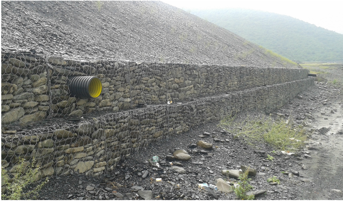
Photo 2. The river embankment in Kvareli
