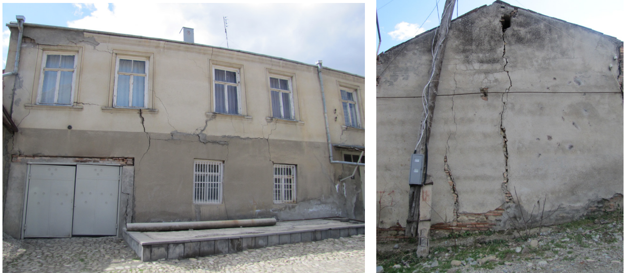
Fig. 2. Damaged buildings and premises
