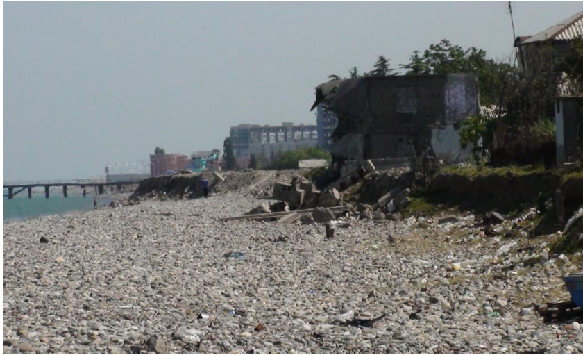
Photo. 1. Destroyed house by sea in the village Adlia
