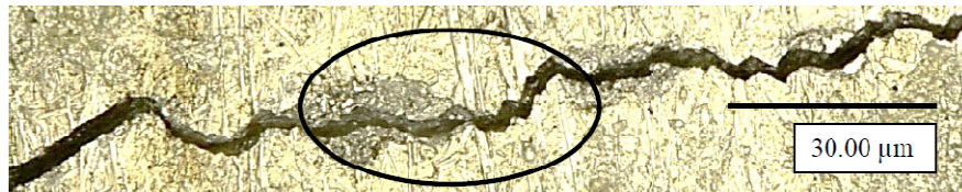
Figure 15. Close up view of a crack on the aluminium panel section showing possible debris (circled) after plasma paint stripping.
