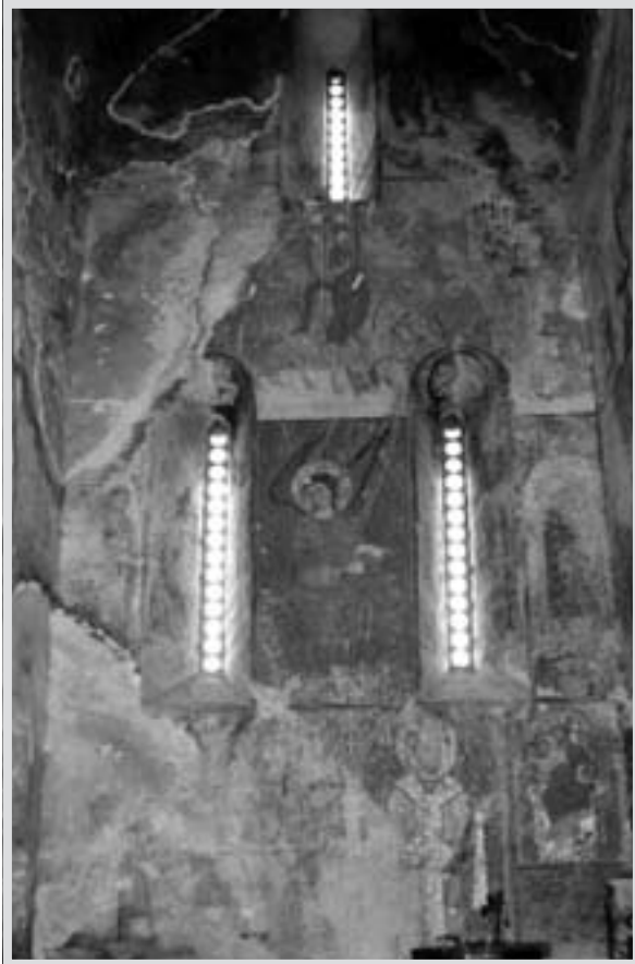
1 Transept at Kintsvisi, showing losses, staining of plaster and white fillings.
