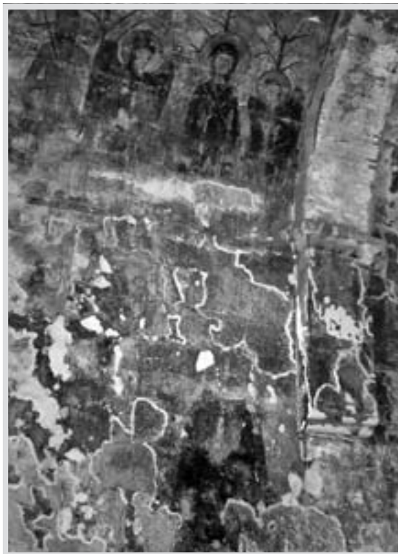
2 Different biodeterioration pattern in the western porch (left with respect to the entrance).
