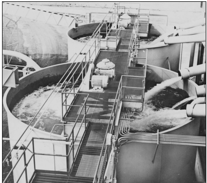
Figure 9. Mechanically-agitated tank for a leaching process
