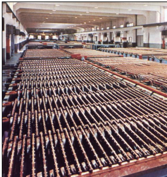
Figure 7. View of a typical electrolytic plant.
